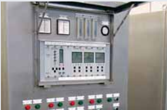
Typical control panel for a MAN Diesel & Turbo process-gas screw compressor unit
