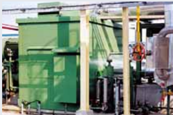
Acoustic enclosure of a process-gas screw compressor unit
