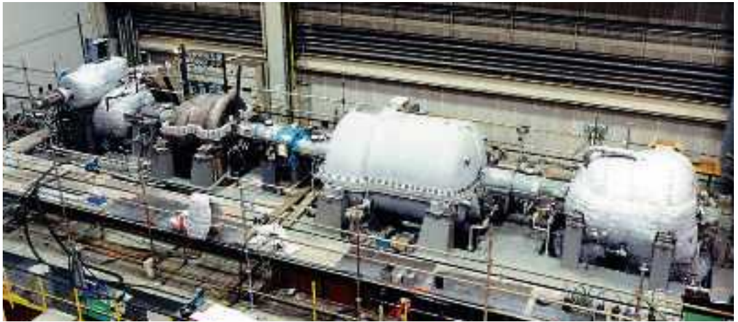
03 Turbomachinery train of a nitric acid plant (dual-pressure process)
